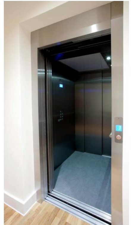
Lift access to all floors
